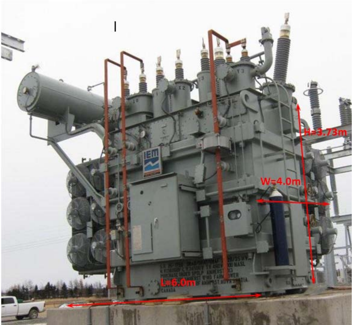
Figure B.2 27.6-kV/115-kVA/30-MVA Substation Transformer
