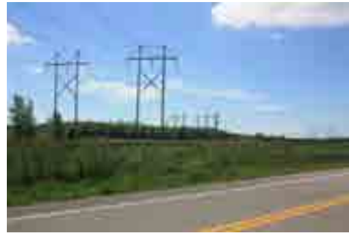
Existing Transmission Line
